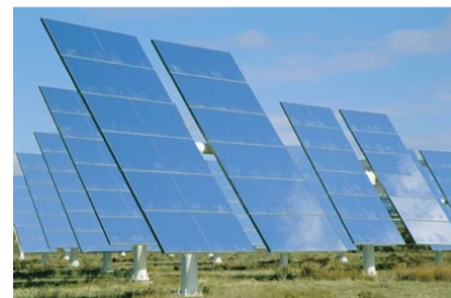
Figure:1 solar photovoltaic panels
