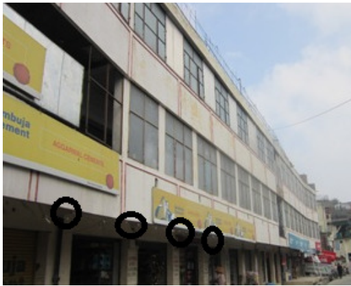
Fig. 9: Cantilever slab loaded heavily
