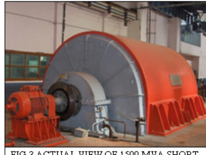
FIG.3 ACTUAL VIEW OF 1500 MVA SHORT CIRCUIT GENERATOR
