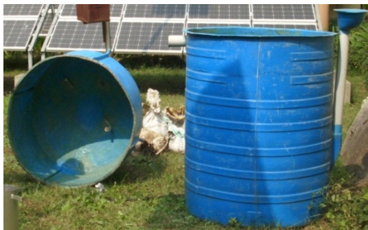
Fig.1: Picture of the biogas digester drums
