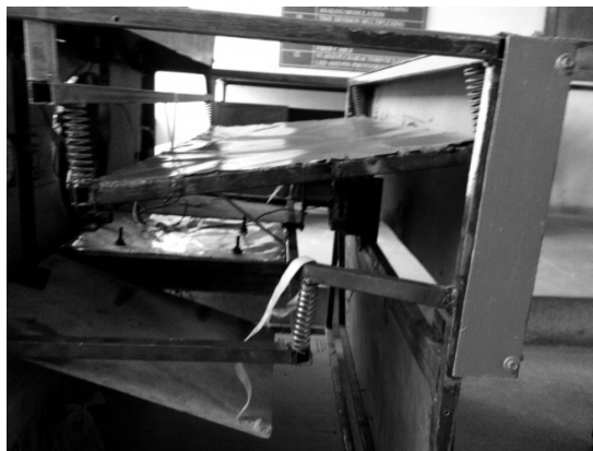
Fig.4. Internal view of IMS bin
